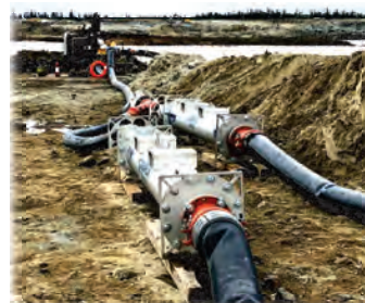
Gold Mine Water Treatment
